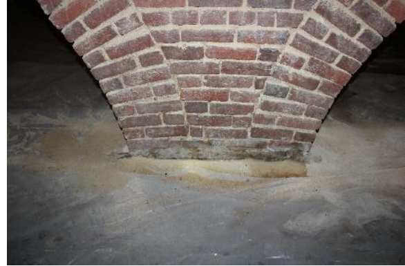
Figure 1.39: Basement, Siege Museum. Note the mortar piled against the base of the arches. (Photograph 7 April 2015)
