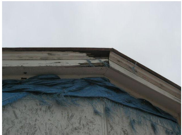
Photo No. 18 Observation – severe wood deterioration at cornice trim.
