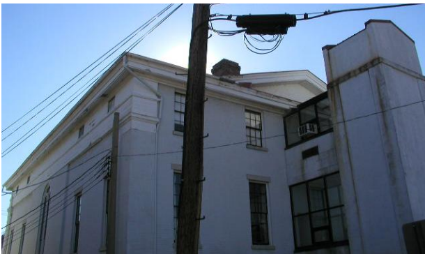
Photo No. 31 Observation – exterior mounted, half round gutter system. Downspout locations - front and rear corners.
