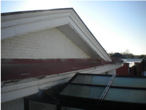
Photo No. 6 Observation –water table area at rear gable. Deteriorated wood trim members noted. Metal cover to be replaced as part of the new roof assembly. Recommend all deteriorated wood trim members to be repaired or replaced and new paint finishes applied.
