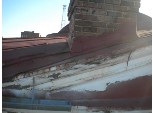
Photo No. 7 Observation of deteriorated conditions at gable trim members. Repairs required. Also modifications to the gutter system noted.
