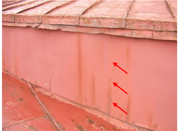
Photo No. 11 Observation of flat wall panels (sheets). Typically nailed into place. Evidence of rust staining also present.
