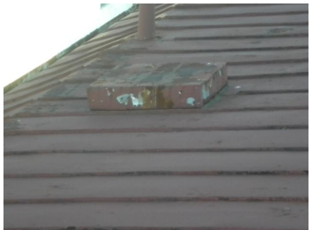
Photo No. 26 Observation – roof access hatch. Deteriorated finishes noted.
