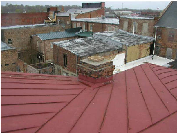
Photo No. 5 General overview on main roof at the rear section. Chimney noted positioned in the valley area.
