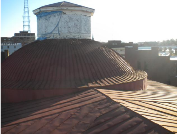
Photo No. 3 General overview of the main roof and dome area. Photo taken at rear section.
