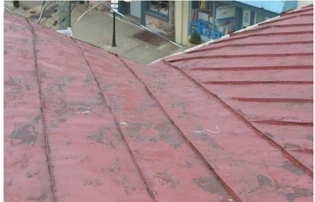
Photo No. 22 Observation – valley area shown. Note position of panels adjacent to the valley.
