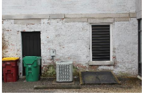
Figure 1.15: North Elevation, Siege Museum. Note the biological growth on the wall and the slope of the asphalt lot sloping toward the building. (Photograph 7 April 2015)
