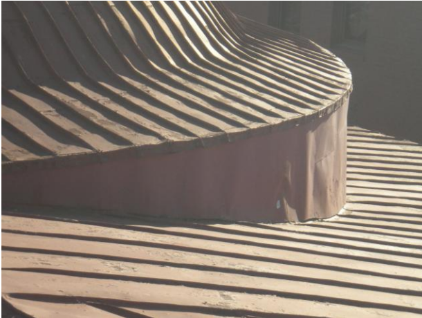
Photo No. 10 General overview of dome structure. Light gauge flat, metal panels observed at vertical section. Standing seam panels observed at dome section with two different slopes noted. Continuous panel lengths conform to the dome shape and are bent to form a drip edge.
