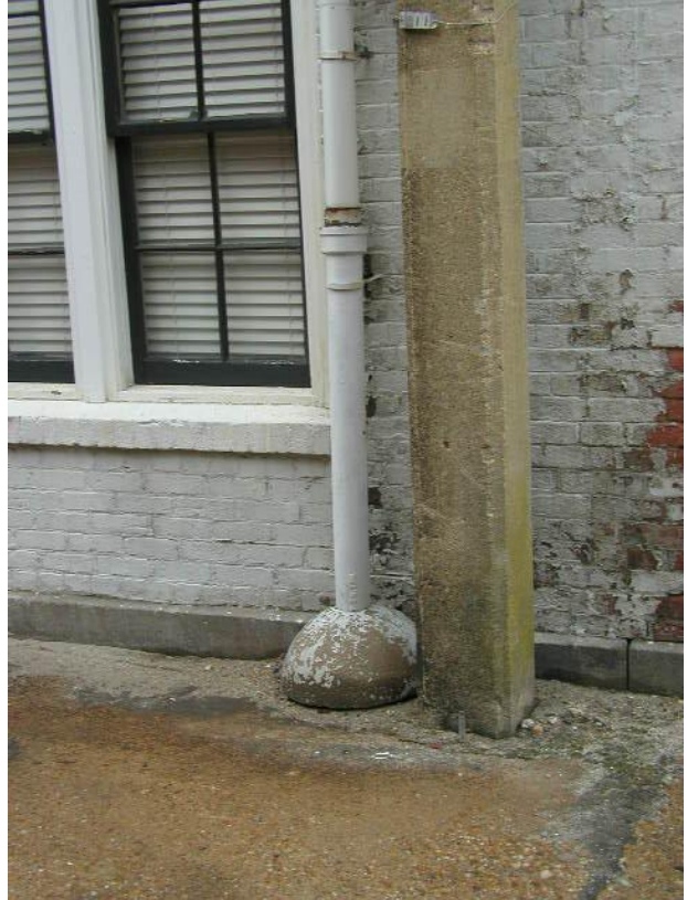
Photo No. 34 Observation – rear corner, east side - downspout routed to cast drain pipe and to below grade storm sewer.
