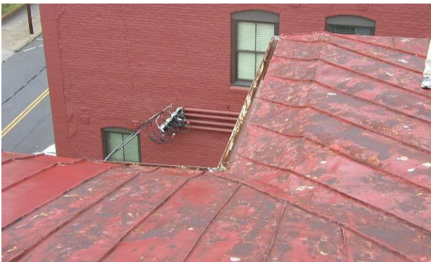
Photo No. 19 Observation at perimeter conditions of main roof area. Transition in roof slope noted. Structural framing below indicates possible built-in gutters at one time. Current gutter conditions shown.
