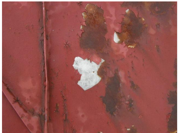
Photo No. 24 Again deteriorated paint finish. The red finish first goes and exposes the tin finish. The tin coating then wears to expose the steel material and rust begins to form.
