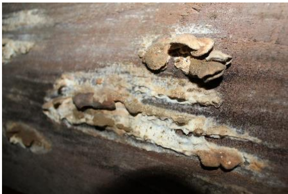
Figure 1.38: Basement, Siege Museum. Biological growth. (Photograph 7 April 2015)
