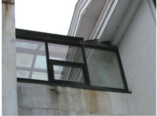
Photo No. 28 Observation – deteriorated conditions noted on stucco finishes. Specific damages noted below window sill area.
