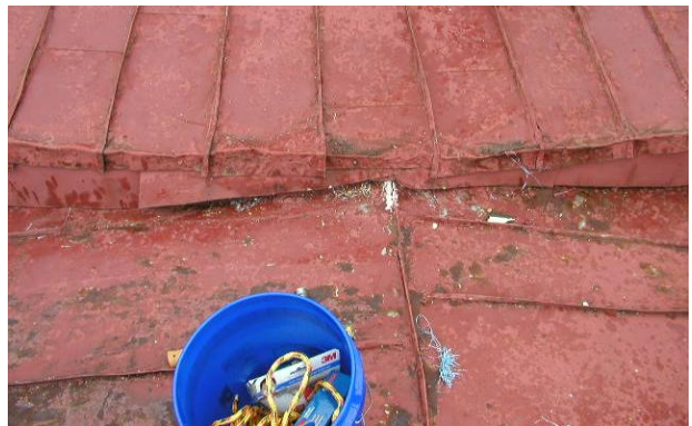
Photo No. 14 Observation of split in metal materials at ridge seam. Solder repair attempt noted.
