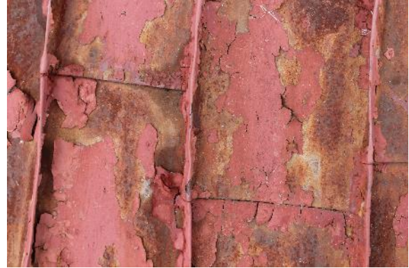
Figure 1.3: Roof, Siege Museum. Detail of roof surface. Note the flaking roof coating and rust beneath. (Photograph 7 April 2015)
