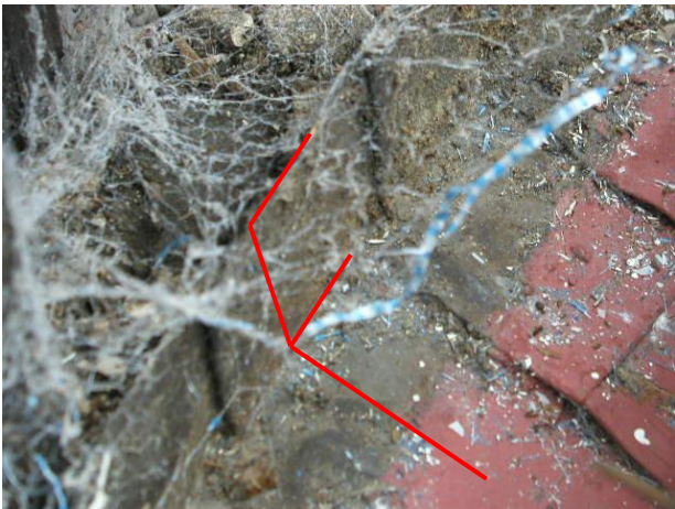
Photo No. 17 Observation – bottom trim board of copula removed to reveal substrate conditions and turned up ends of the standing seam dome roof panels.
