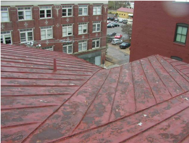
Photo No. 4 General overview of the main area and front portico roof. Valley area shown.
