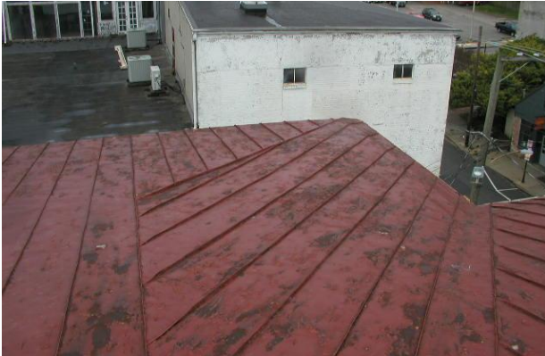
Photo No. 21 Overview of roof slope transitions; slope from ridge to eave, hip detail and valley detail. Panels as installed do not necessarily run parallel to the roof slope. Configurations exist where damming conditions are created and water is forced to run across the standing seams.
