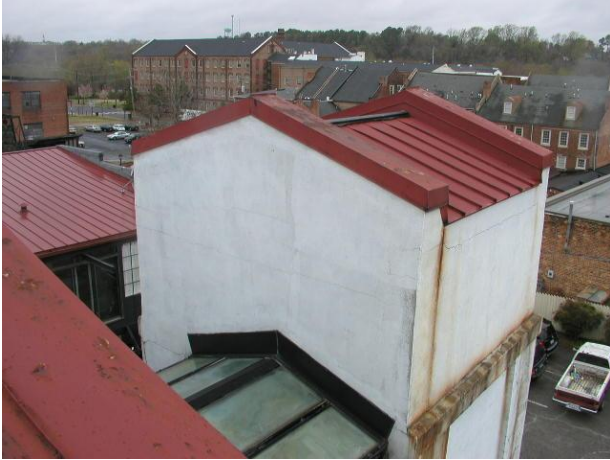
Photo No. 27 General overview of elevator roof area. Similar standing seam panels noted. Also metal coping covers. Deterioration noted on paint finishes. A Retro-fit ridge cover has been added.
