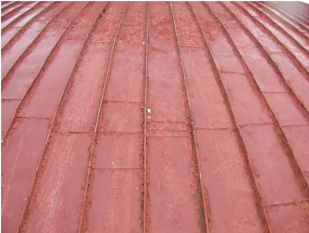
Photo No. 12 Observation - panel runs are fabricated from various lengths of the sheet material and have numerous lap seams. Note the width of the panels. Pans start out at a minimal width at the base and taper to a fairly narrow width at the top of the run.
