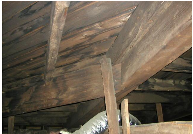
Photo No. 9 General observation of underside of roof deck. Typically dry. Water stains noted on wood components. Reference the structural section of this report for further discussion.
