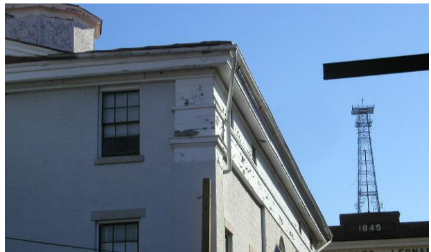
Photo No. 32 Observation – exterior mounted, half round gutter system. Downspout locations - front and rear corners.
