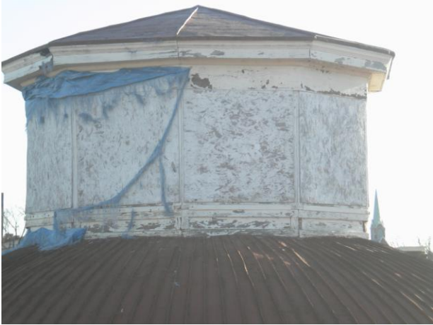
Photo No. 15 Observation of cupola or lantern. Deteriorated wood conditions noted at cornice area and at base. Flat seam panels noted at roof area.
