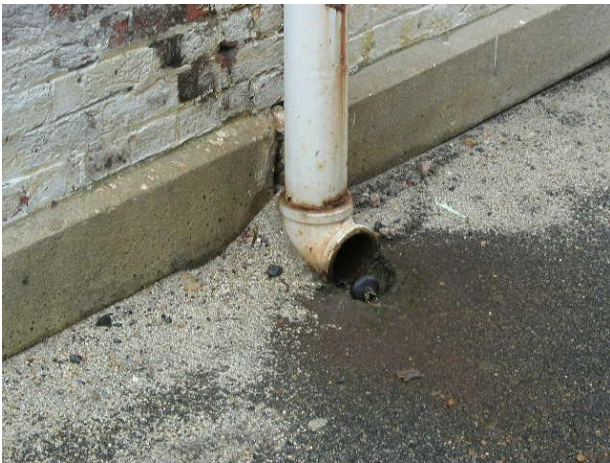
Photo No. 35 Observation – rear corner, west side - downspout routed to cast drain pipe and discharge at grade.
