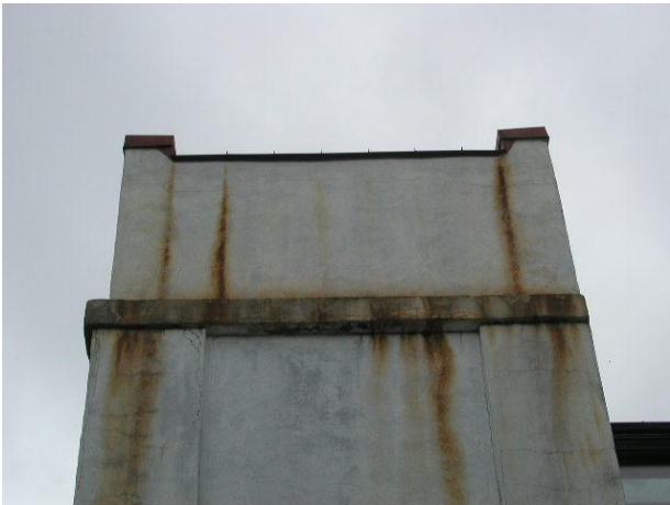
Photo No. 29 Observation – rust stains noted on stucco wall finish.
