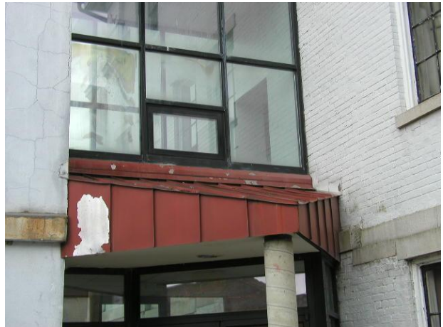
Photo No. 30 Observation – small roof area at rear entrance. Deteriorated finishes noted on the metal components.
