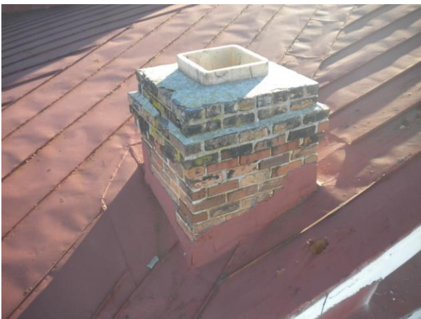
Photo No. 25 General overview of chimney. Located in valley area. Some repairs noted.
