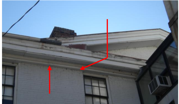
Photo No. 8 General overview of area as discussed in photos no. 6 & 7. As part of the roof renovation, recommend new paint and wood repair down to the brick line as a minimum.
